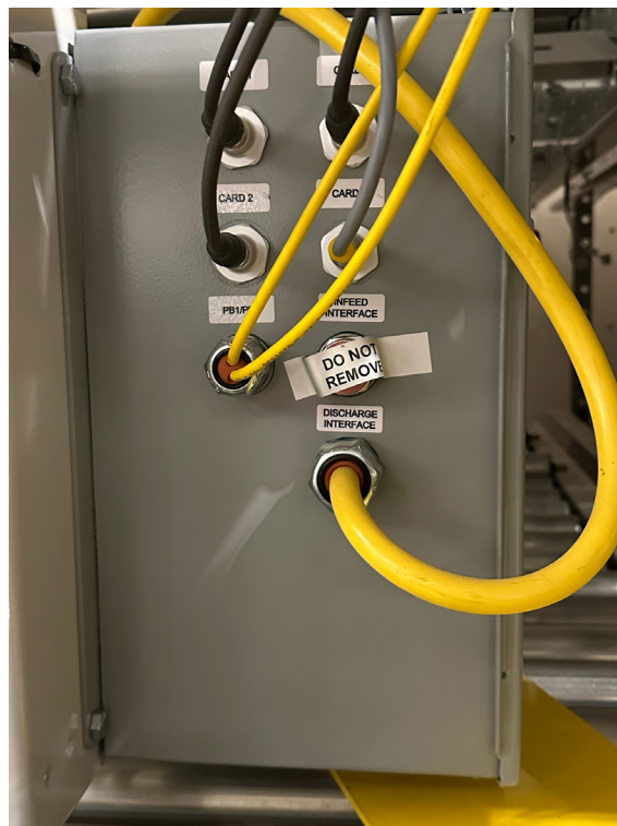
Figure 1: Master panel with Infeed Interface covered with tamper resistant sticker.
