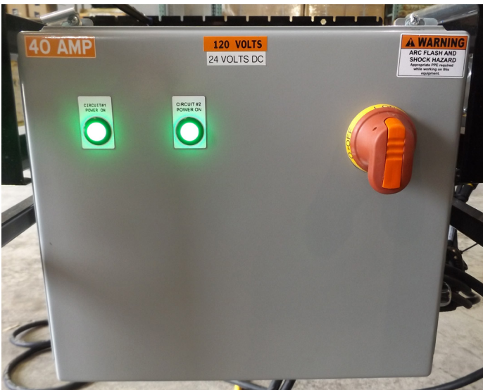
Figure 28: 40 amp Power Supply with power applied during normal operation.
