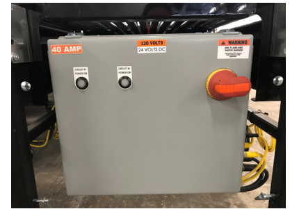
Figure 7: Power Panel with Disconnect Switch
